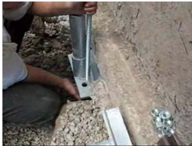
Fig. 2. Underpinning arrangement with vertical piles without cutting off the footing projection (RS).
