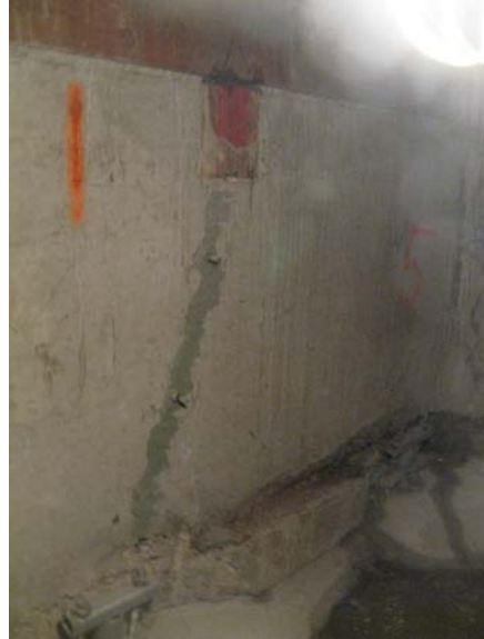
Fig. 5. Reopening of previously epoxy-injected crack due to bending of anchors caused by upper soil saturation from a plumbing leak (Case Study 2).
